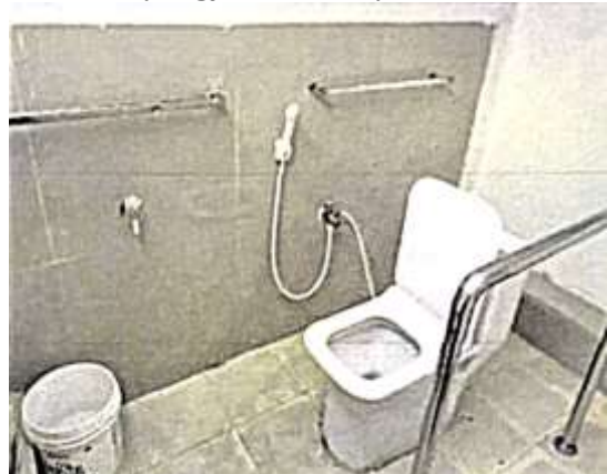
Divyangjan Friendly Bathroom
